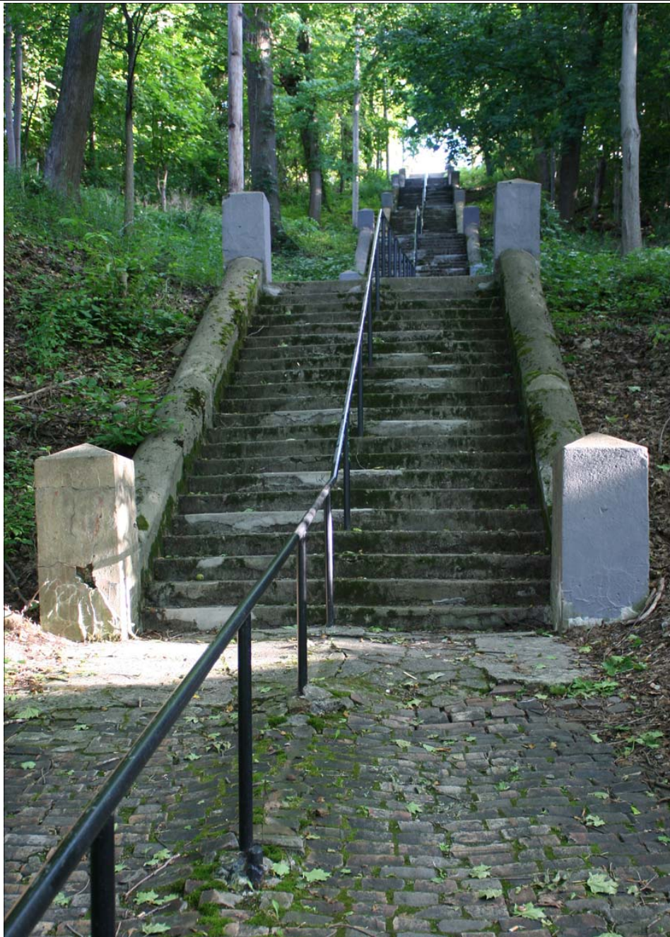
SEUNA led efforts last year to address the poor condition of the Westminster Steps. As a result, the city replaced the center handrail from top to bottom and many of the concrete steps have been repaired. Obviously, there is still work to be done.
